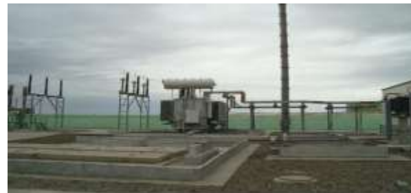
Cement plant substation
